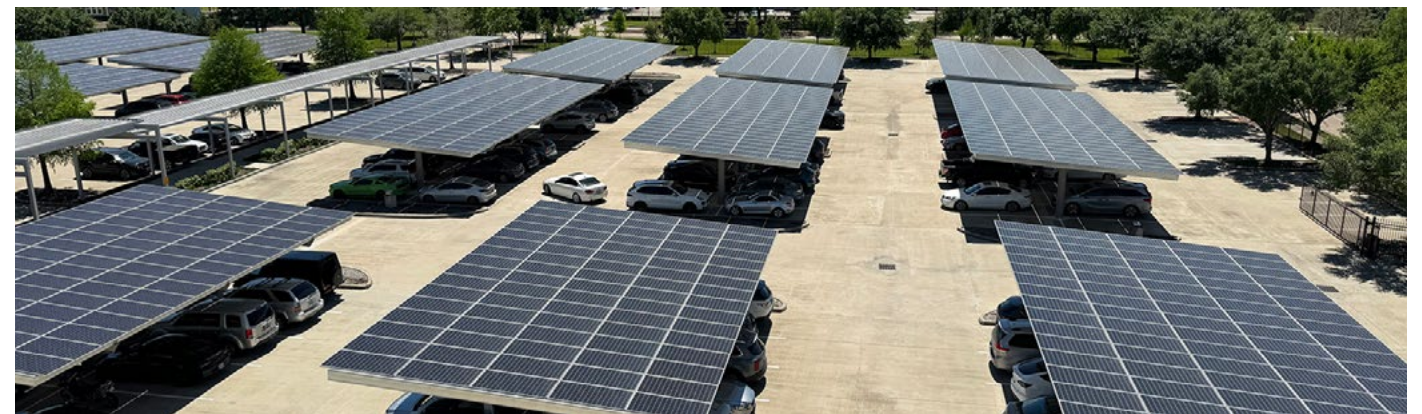
The TGS Houston Operational Headquarters landmark solar energy parking canopy in Houston, Texas. Consisting of 1,700 modules, the installation is projected to boast an annual output of 929,034-kilowatt hours of energy – creating a unique approach to achieving the Company’s net-zero targets.
