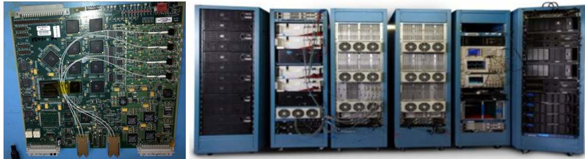
Figure 3 Optical demodulator and complete optoelectronic system that was installed on the Jubarte P57 FPSO. Left to right, UPS battery backup rack, laser rack, (2) optoelectronic racks, Test equipment rack and data acquisition and storage rack.
